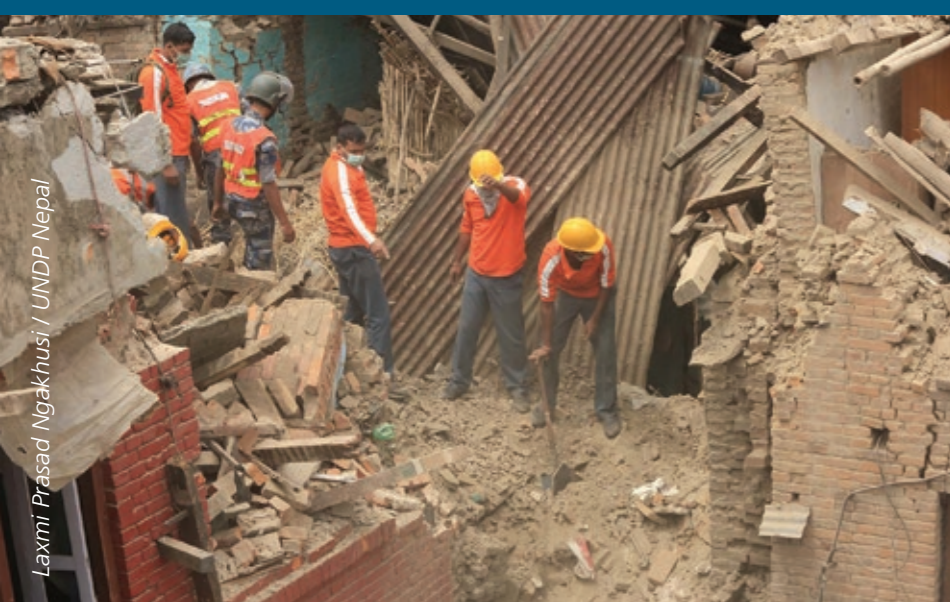
Some of the damage in Bhaktapur.
