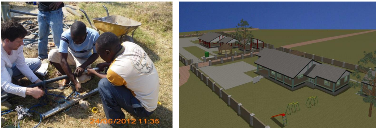
Figure 3 Repairing a borehole at Kaoma orphanage in Zambia (left) and a 3D model of planned project for the orphanage (right).
